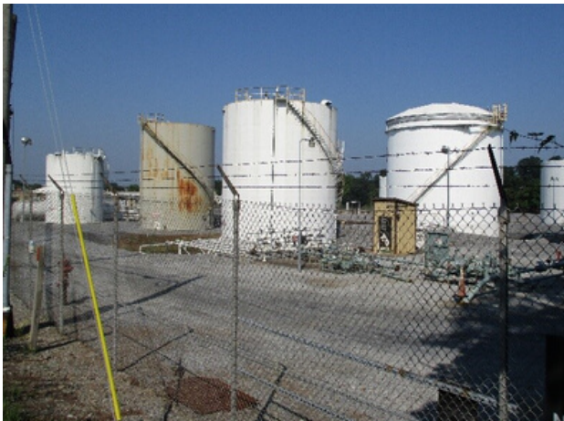
Above ground storage tanks at project petroleum distribution facility site.
