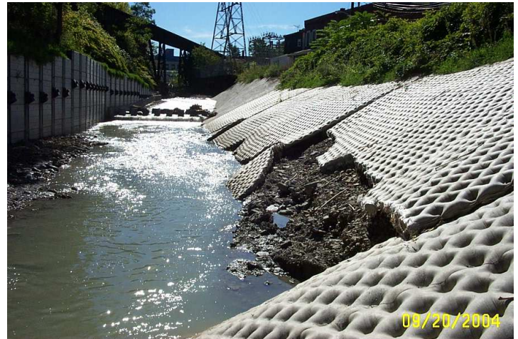
This photo taken by the Corps shows the revetment mattress after Hurricane Ivan flooded the area. The recent channel improvement held up remarkably well considering that this was the second major flooding event in a one week time frame.
